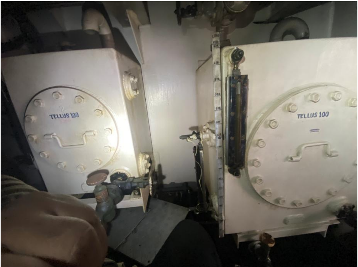
110. Hydraulic storage tanks in steering gear room.
