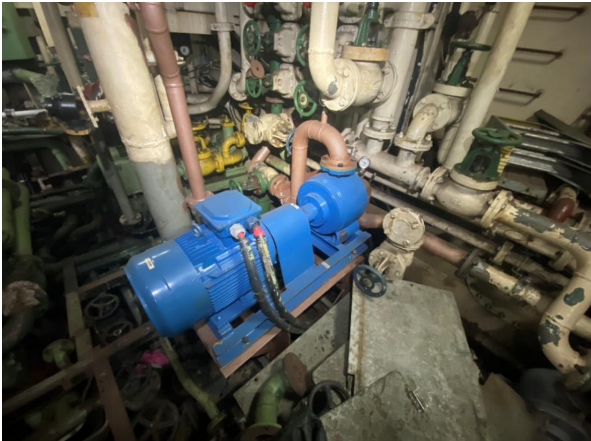
082. Newly installed pump and motor, likely for seawater system.
