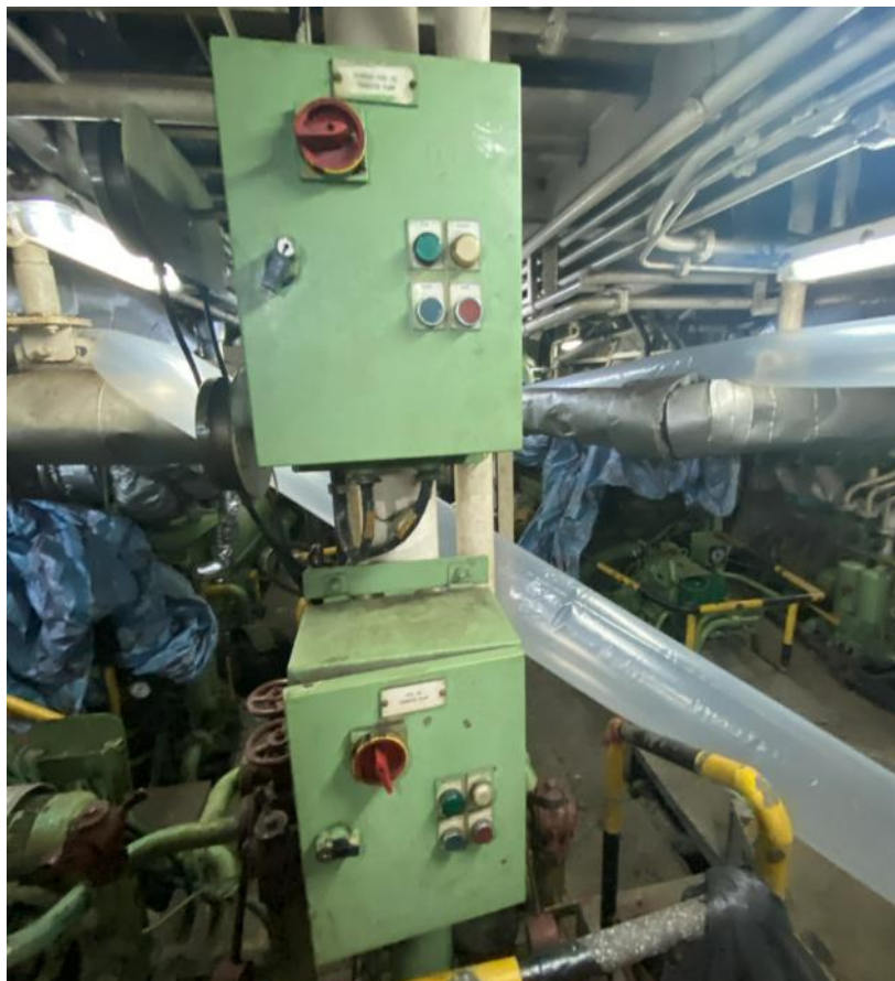
092. Fuel transfer pump control panels.
