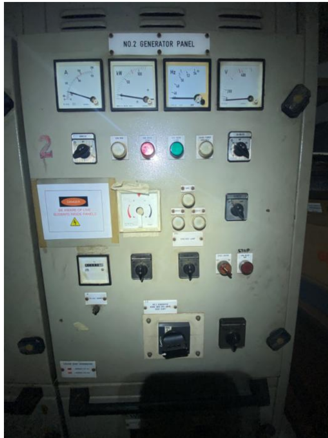
099. Generator engine switchboard.
