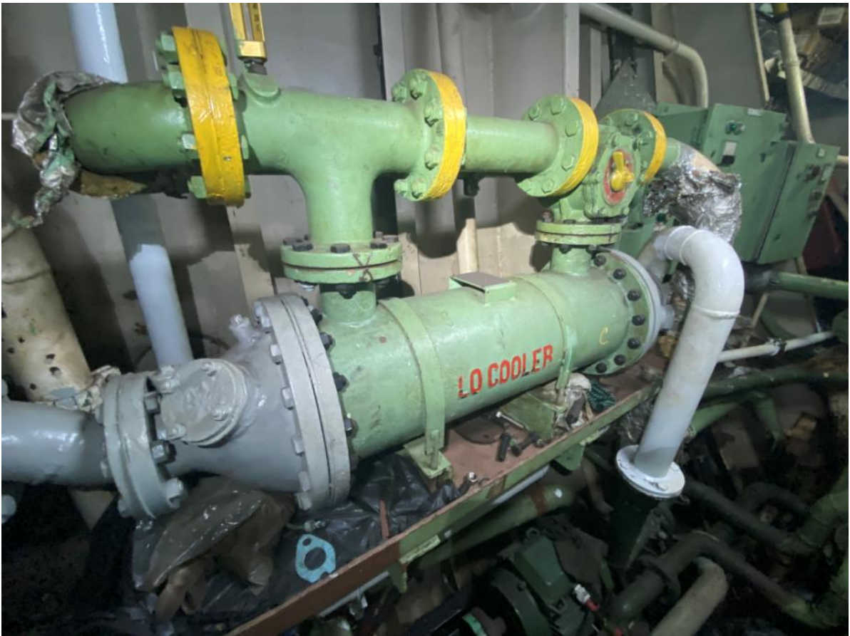
087. Portside main engine cooler.
