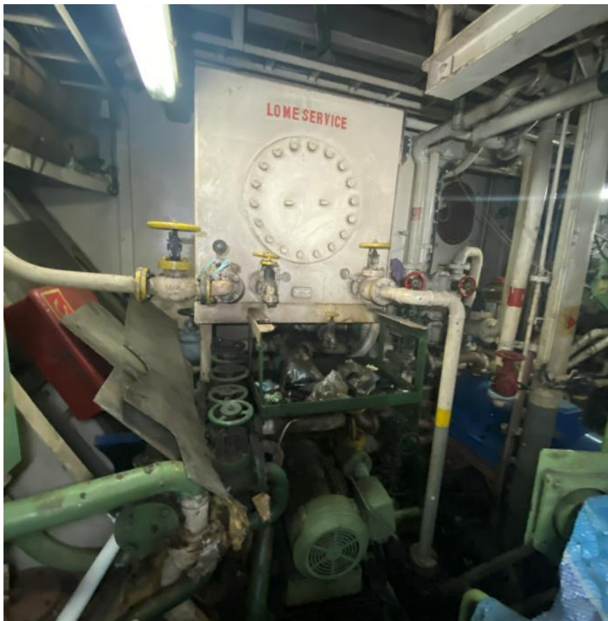
086. Main engine lubricating oil service tank.
