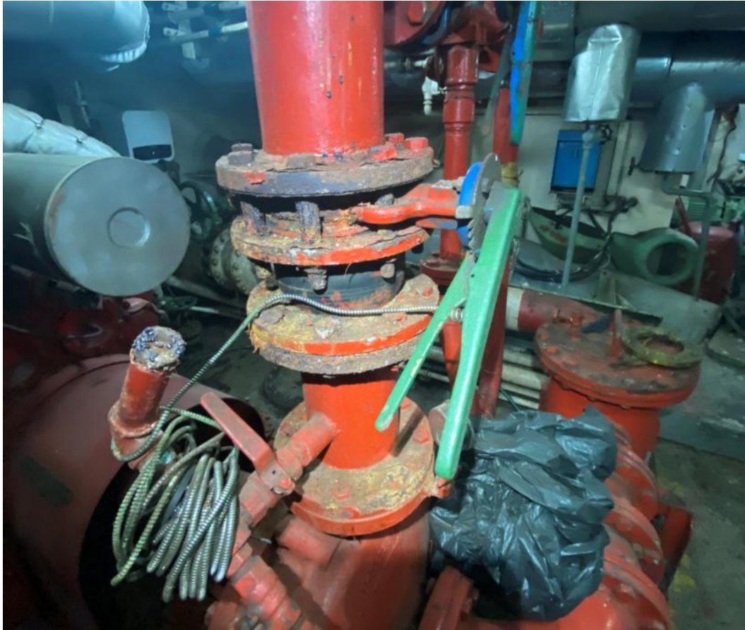
095. Corrosion in way of FIFI pump outlet valve.
