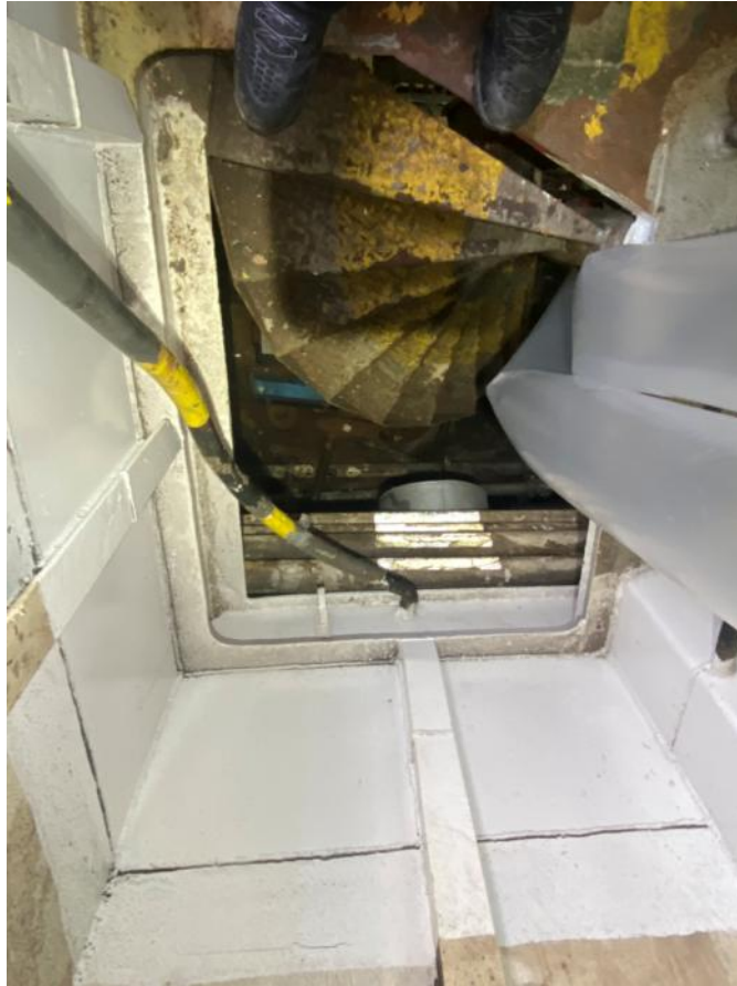
071. Spiral stairs into engine room.
