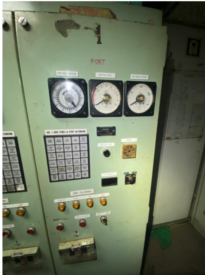
101. Main engine alarm and indicator panel.
