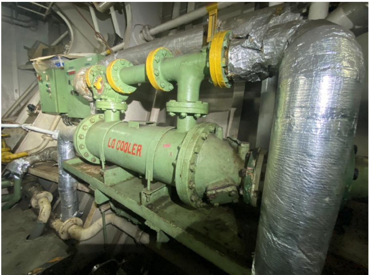
076. Starboard engine cooler.
