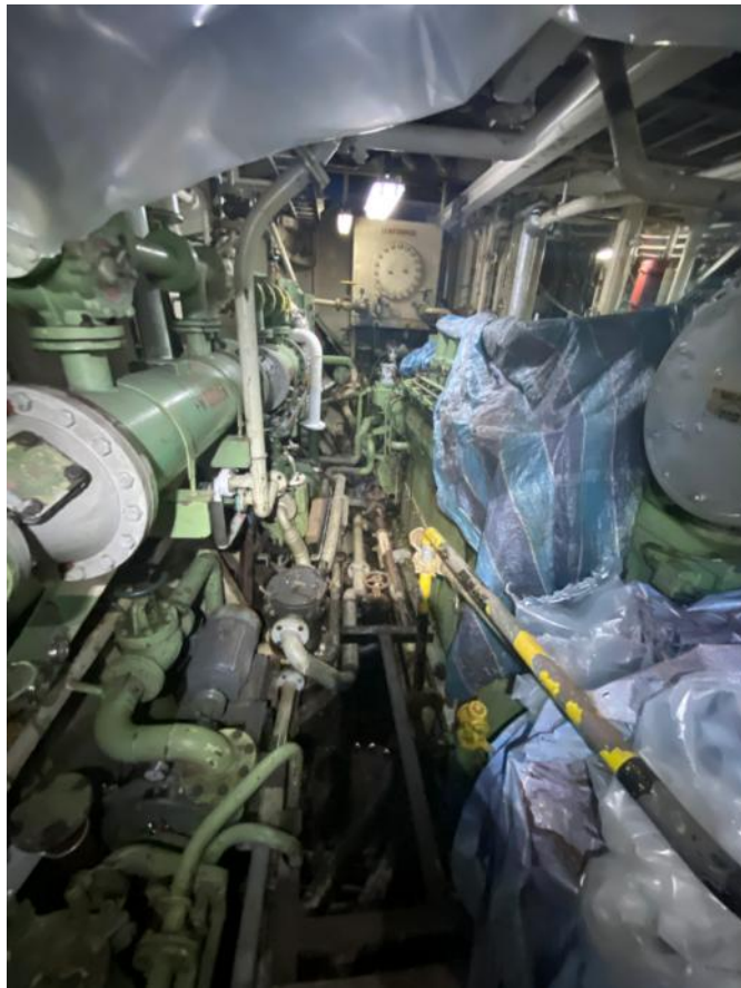
090. Portside of engine room.
