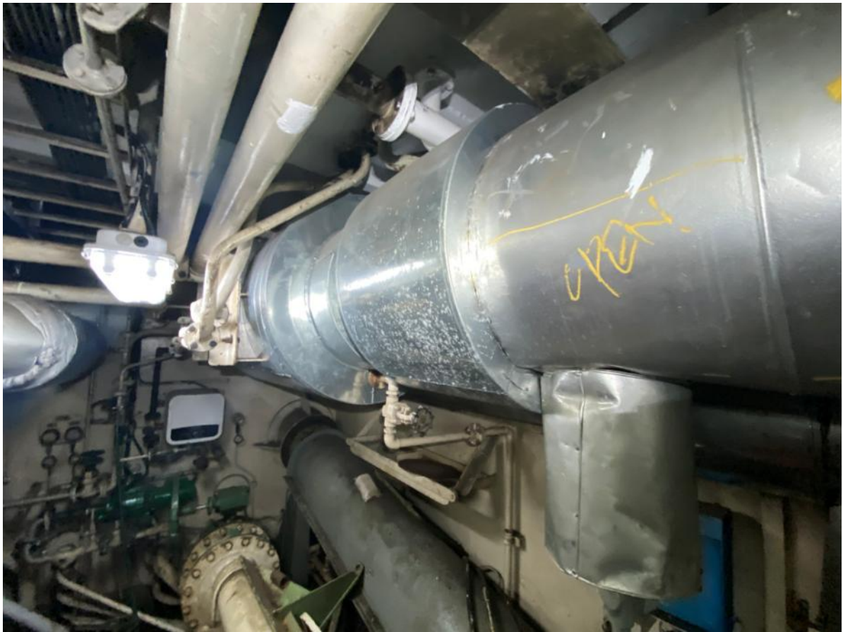
097. Exhaust insulation covers appeared new.
