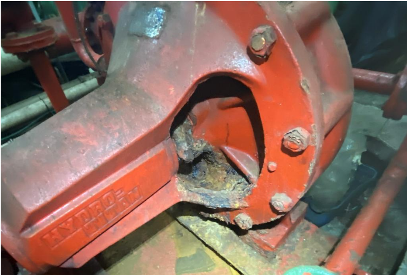
094. Corrosion found in way of pump casing.
