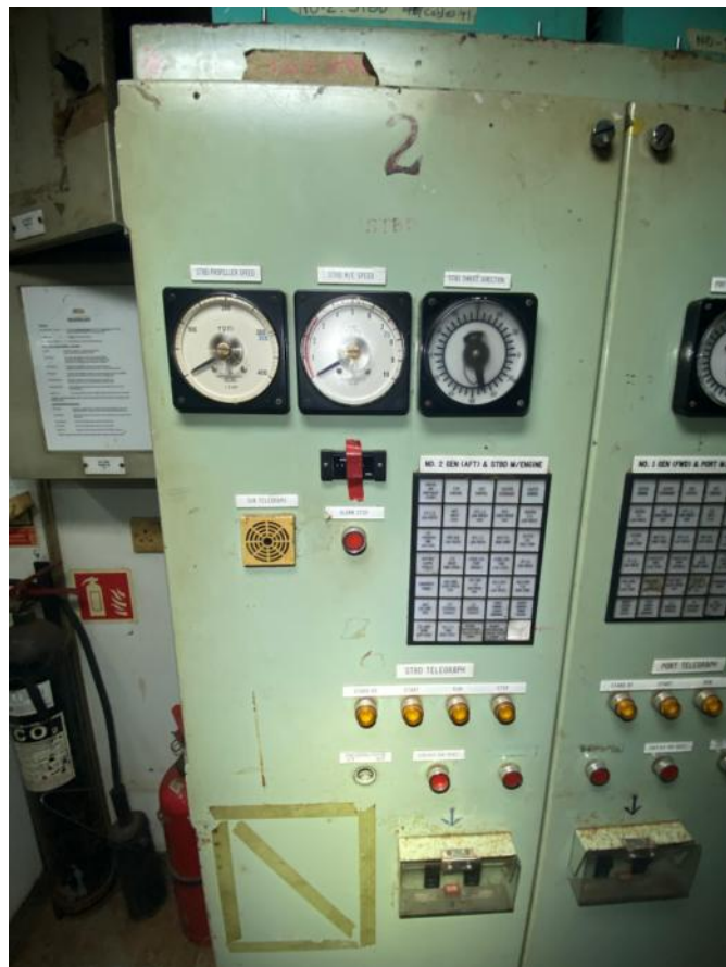
102. Main engine alarm and indicator panel.
