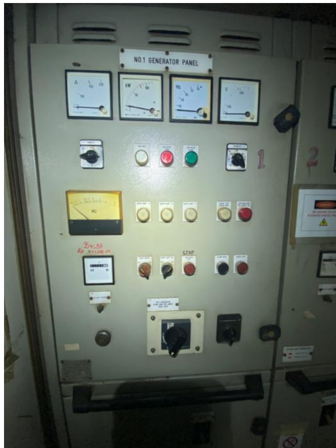
098. Generator engine switchboard.
