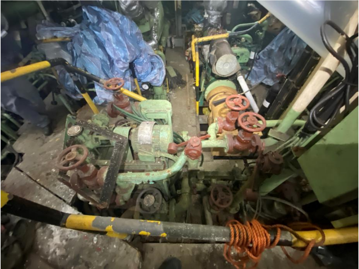
091. 2 nos. fuel transfer pumps.
