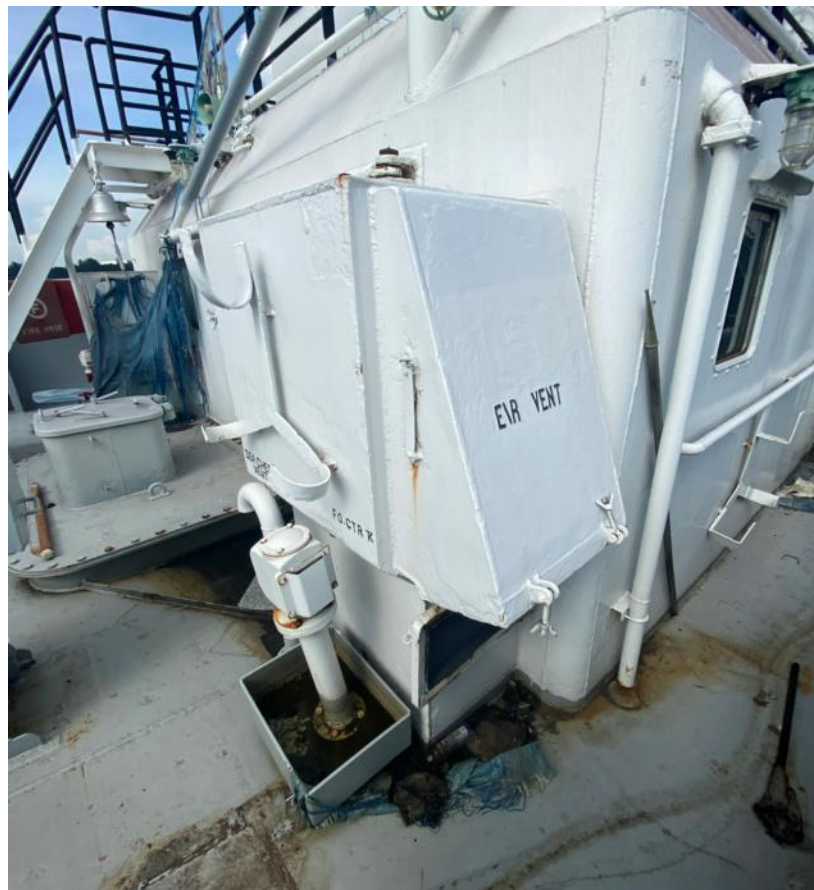
018. Engine room vent.
